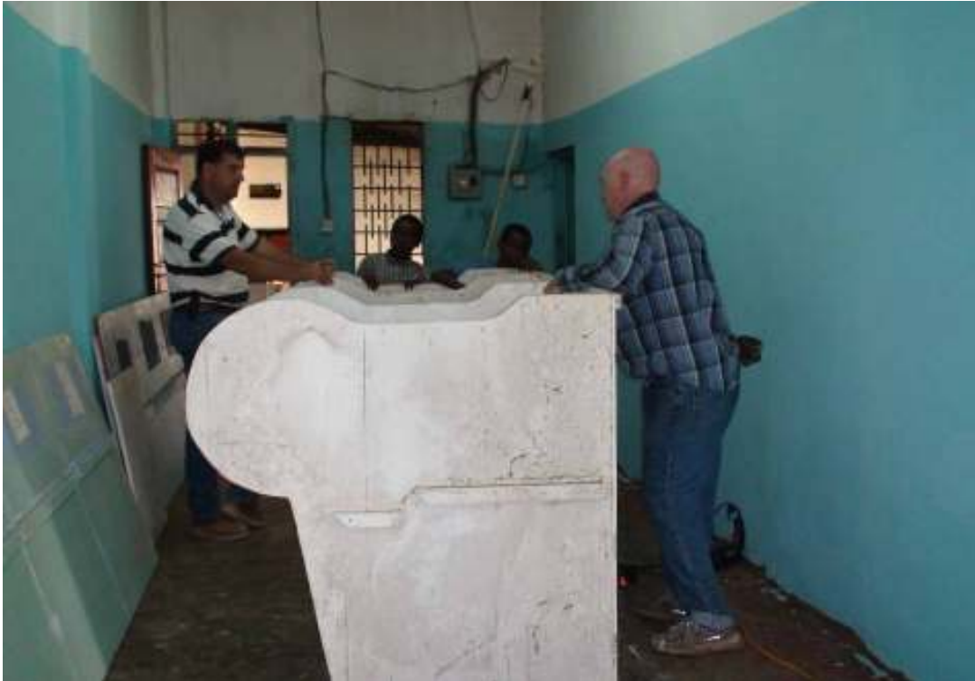
Bro. Mike McMillan and Bro. Jeff Ruegsegger assembling and installing desks shipped from America in a section of the old boy's dorm that will be our new school.
