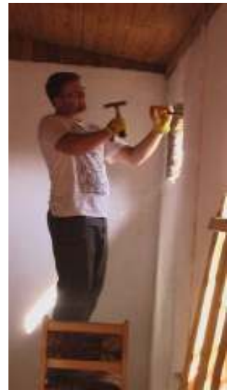
Bro. Kirk making an air conditioner opening in the new orphanage apartment.
